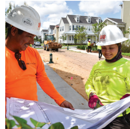
Construction Foreman Roberto Lara and team member Dayana Chacon working together at the Celebration Island Village project.
