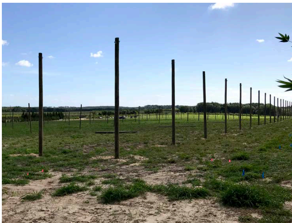
The CUPS structure under construction in Groveland. CUPS creates a more controlled environment where citrus groves can be grown with fewer pests and diseases.
